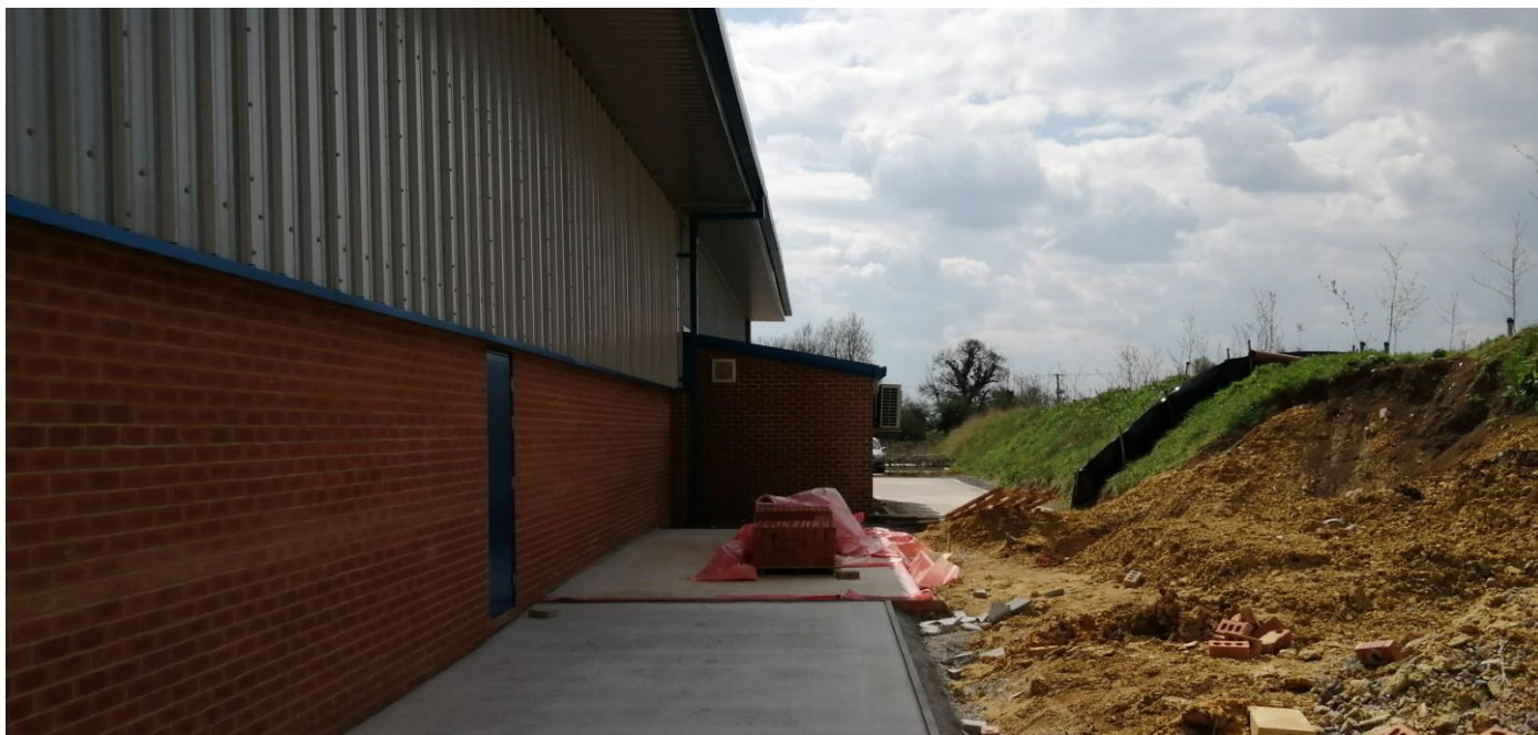
View of the western end extension of unit 8 and unit 9's existing lean to extension
